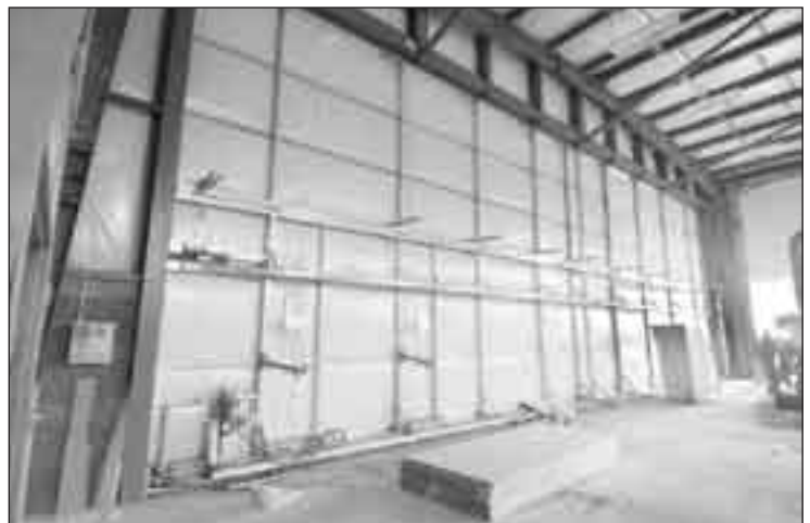
Helicopter access to the hangar will be through a 60- by 20-foot clamshell, aluminum door.
