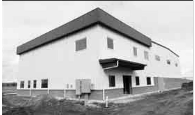
Winco Helicopters will soon move into its new headquarters at the Aurora State Airport in Marion County. The company chose a custom designed and engineered, steel-frame building that is being built by Portland general contractor Engineered Structures Inc.
