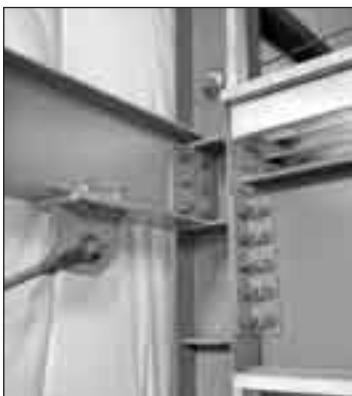
Thanks to excellent design, engineering, and fabrication, buildings like Winco's headquarters are strong, efficient, and easy to build.
