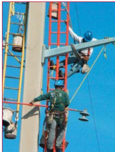
Once in proper position, the bells are secured and the crew is ready to move to the next set of bells or the next structure.
