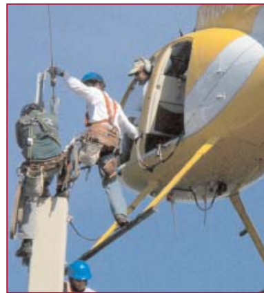
Once the crew reaches the next pole, they are dropped off to start replacements of the bells on each davit arm.
