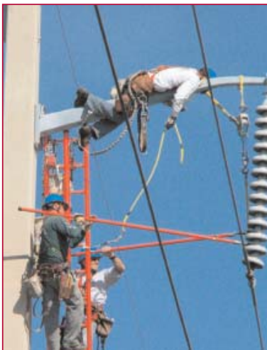
The potentially faulty bells are removed and the equipment is prepared for the addition of the new bells.
