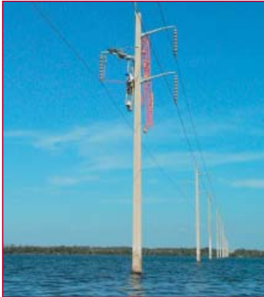
The project at the Matlacha water crossing entailed replacement of bells on 25 poles as well as a cross-arm replacement.
